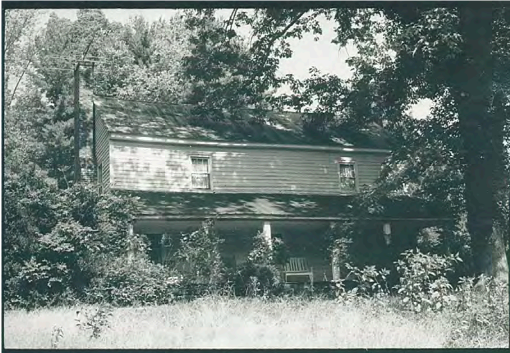
Facade of the John Shroat House. Documentary photo from the North Carolina State Historic Preservation Office survey file (1980)
