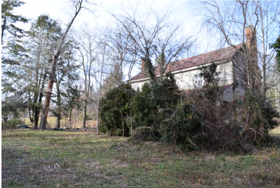
Facade of John Shroat House obscured by vegetation, view to the northwest
